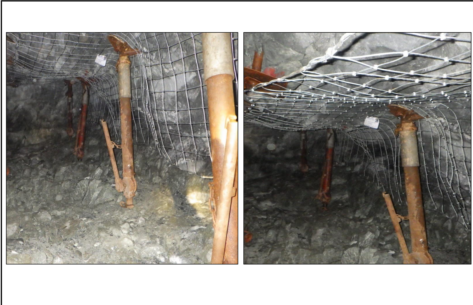
Photos taken on the 23-09-2022 – New Start up panel (First Safety Net)
