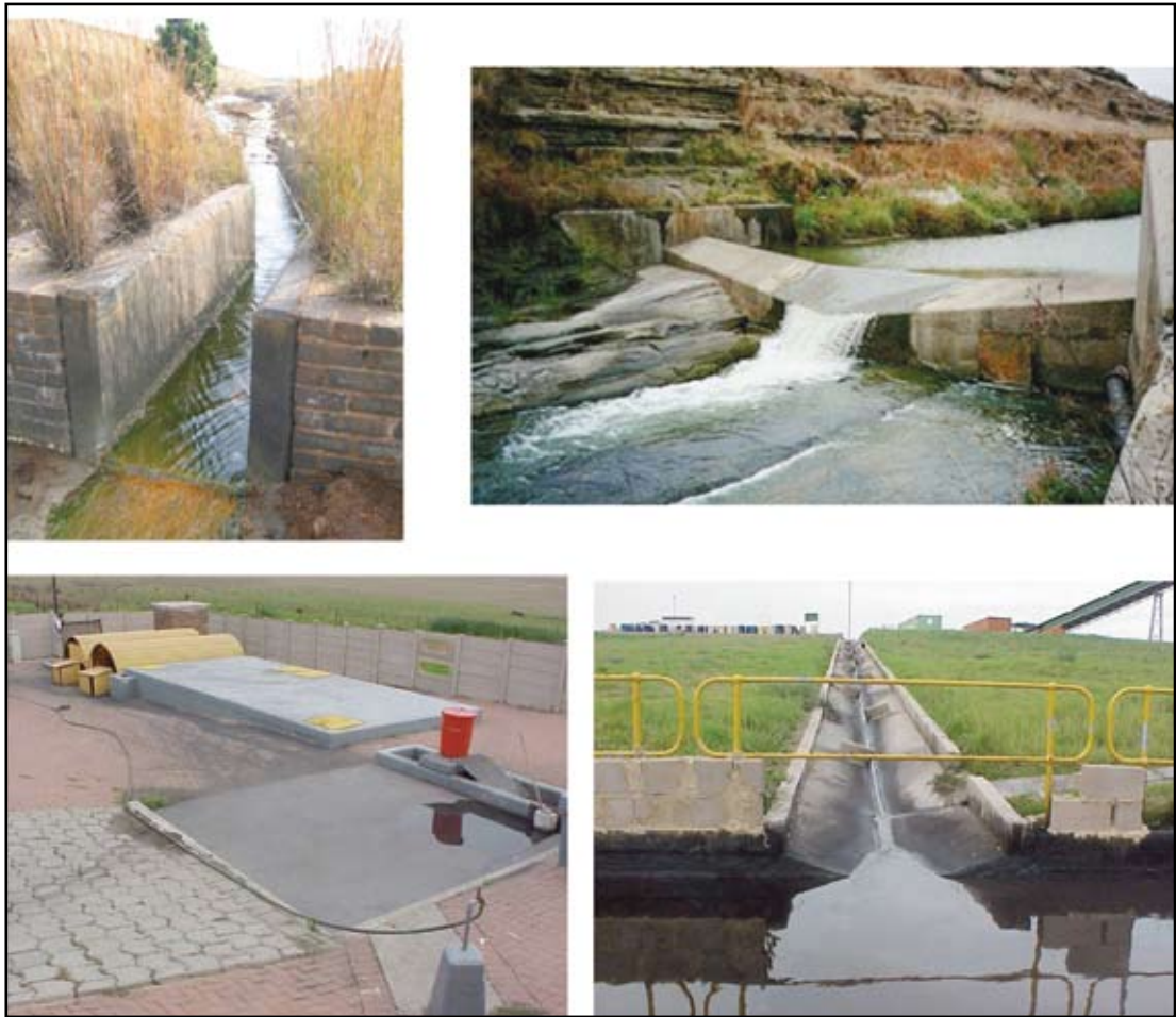
Figure 6-23: Examples of well maintained water management systems
