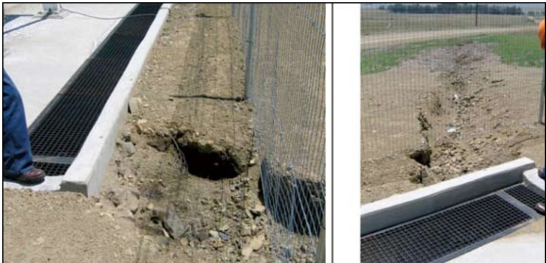
Figure 6-6: Example of poor water separation practices
