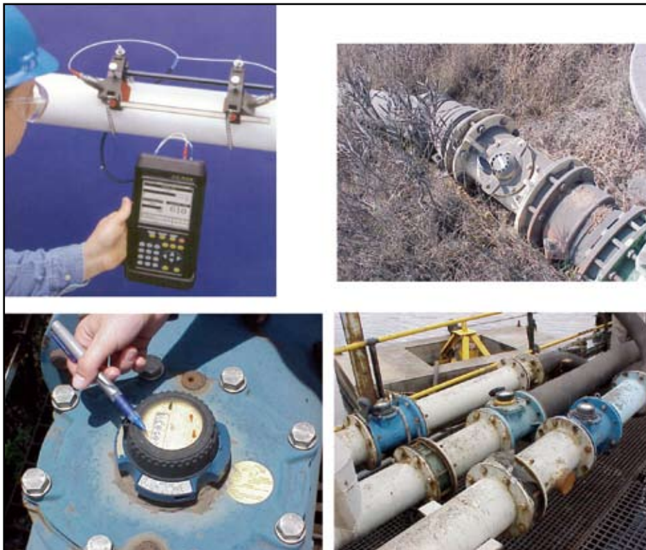
Figure 6-30: Pipe flow monitoring
