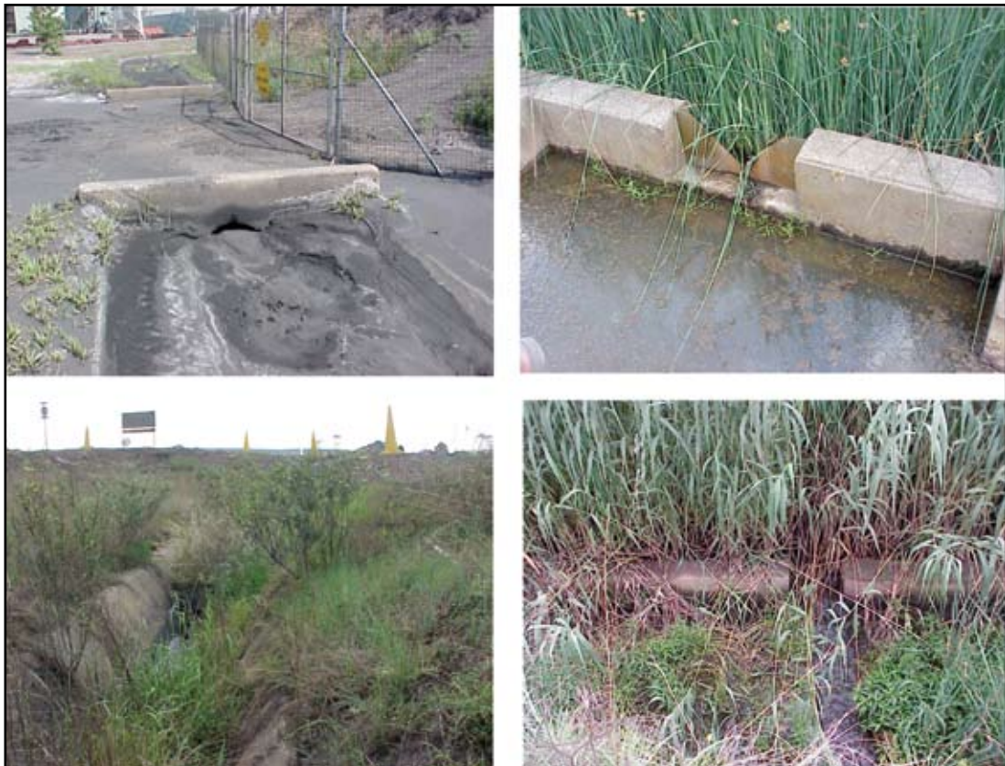
Figure 6-24: Examples of poorly maintained water management systems
