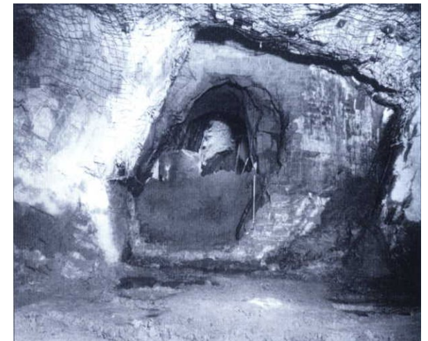
Failed backfill bulkheads
