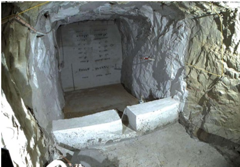
Concrete water retaining plugs
