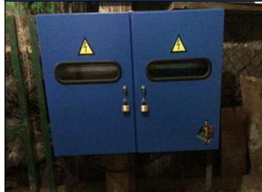
Charging cabinet is installed in central waiting place
